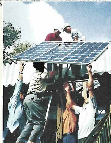
THE SOLAR ELECTRIC LIGHT FUND (SELF), which received a grant from the RBF in 1996, conducts grassroots solar home electrification projects in China (top) and Vietnam (bottom), among other developing countries.
